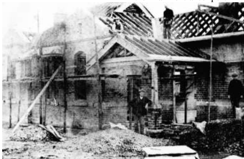
Station being built in 1912, Joe Kidd, foreman builder for Alf Frongerud in foreground
